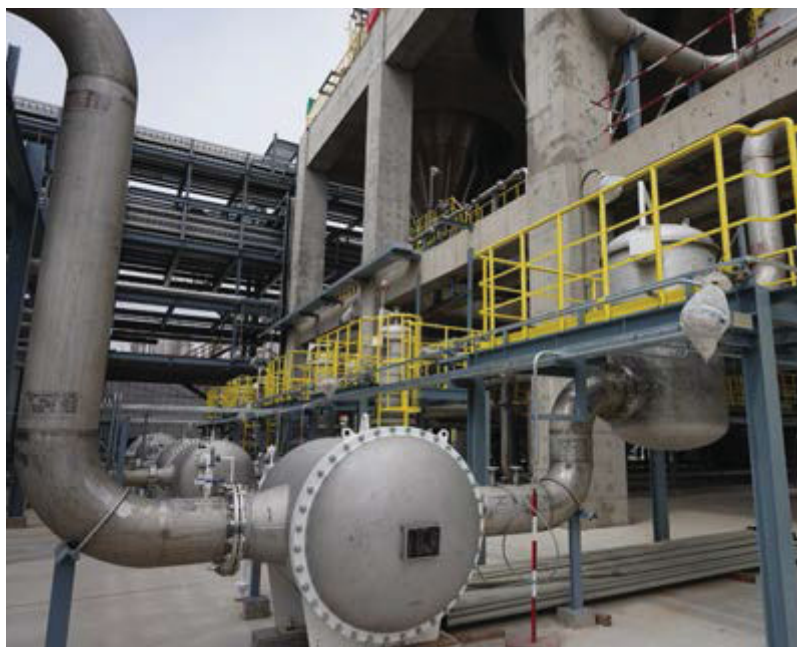
FieldComm Group's technologies are the basis of the plant's improved operations, maintenance and asset productivity. Source: Wanhua Chemical Group
