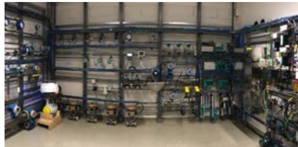
Figure 1: To evaluate Ethernet-APL networking, communications and devices via Profinet protocol, BASF built a field test lab in 2019-20 at its headquarters in Ludwigshafen, Germany. The lab tests flowmeters, level, pressure and temperature transmitters, valve positioners, sensor sets, and other components, which is helping its supplier partners develop Ethernet-APL products. Source: BASF
