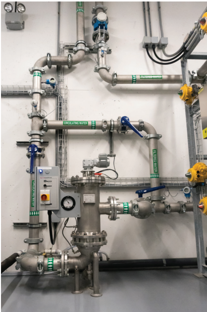
FIGURE 3. This smart pumping application in UV disinfection uses smart instruments to monitor flow control and pump speed to ensure water is passing through the system at precise rates to guarantee quality.
