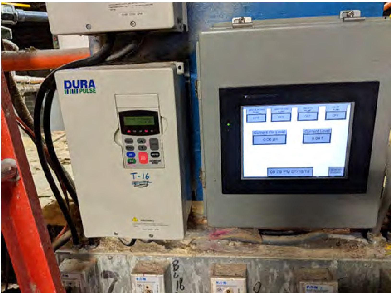
Figure 8J: HMI: An AutomationDirect C-more EA9 Series 15-inch touch panel HMI was added to the new control system to provide status, data trending, historical data, reporting and other functions.
