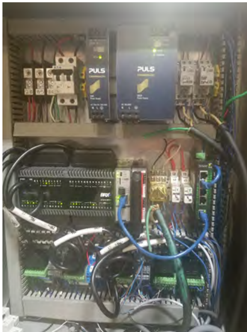
Figure 8i: Control Panel: This new AutomationDirect BRX PLC replaced the existing Click controller with minimal required changes or wiring additions.
