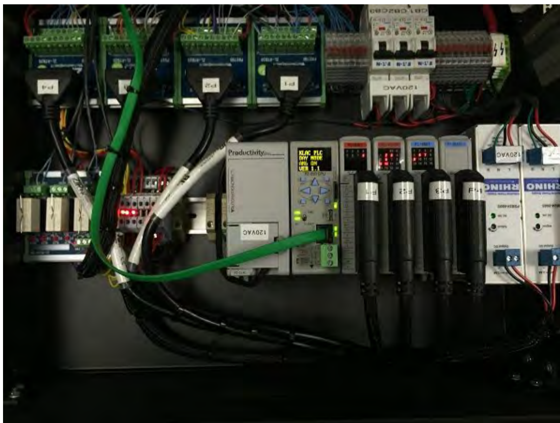
Figure 8B: An AutomationDirect Productivity2000 PLC was used to automate transmitter pattern and backup switching at a remote facility.
